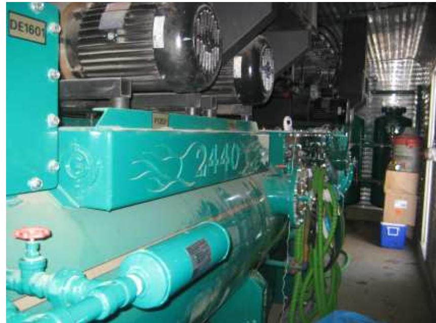
DPVE treatment system in Lions Park.
